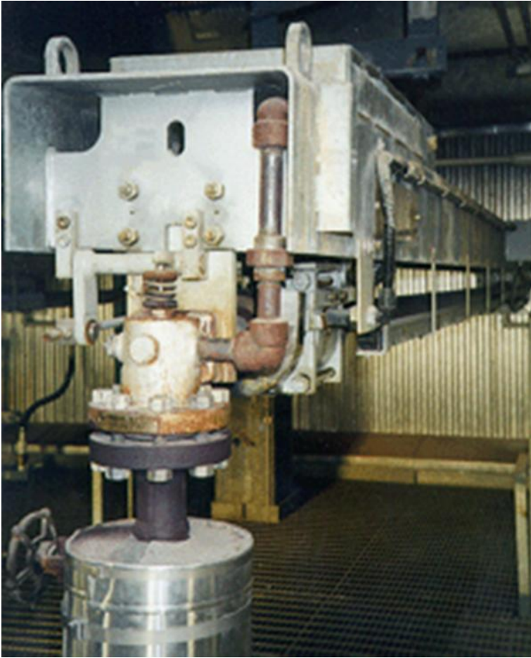
Figure 5 – Recovery Boiler Sootblower
